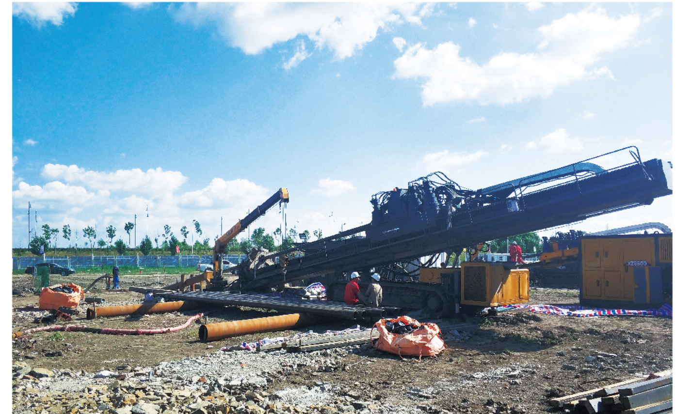
XZ6600 working for the 3 km water supply pipe project with a diameter of 813 mm across the Songhua River
