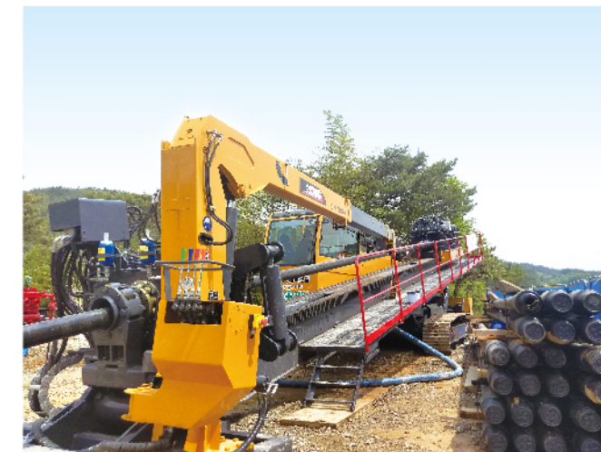
XZ3600 working for water supply pipeline hard rock construction in South Korea
