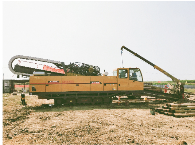
XZ3600 working for the construction of 1346 m long pipeline, with a diameter of 717 mm, in Shandong
