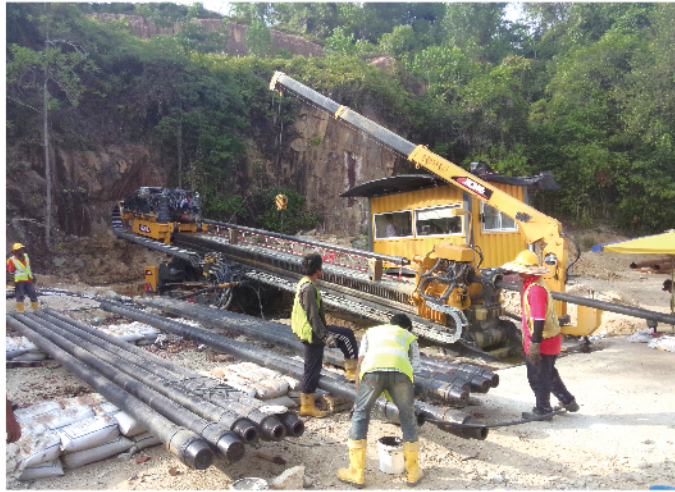
XZ5000 working for the construction of power pipeline crossing gulf in Malaysia
