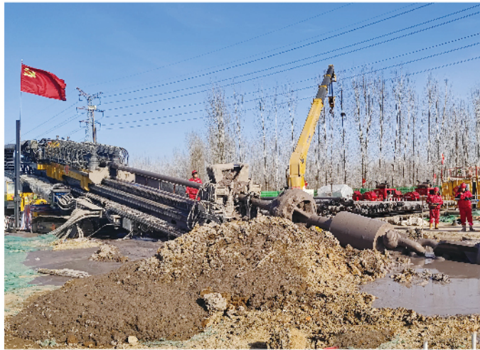
XZ13600 working for the construction of 1334.8 m long pipeline, with a diameter of 1219 mm, in rock stratum
